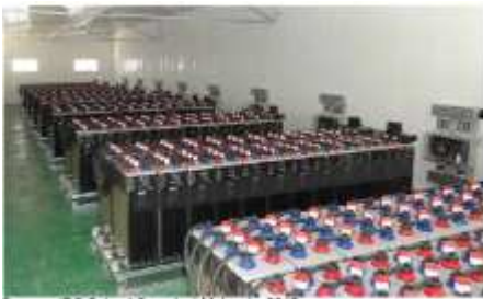
Source: IBC Solar AG, project Malaysia, 2012
